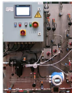
②Dosing unit and SCR control panel
