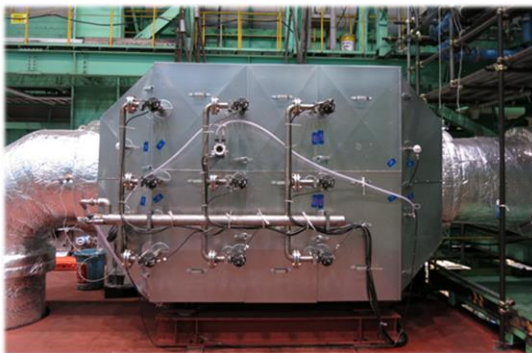
①SCR Reactor with Soot blower
